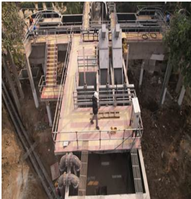
55 MLD STP at Assi BHU, Varanasi
