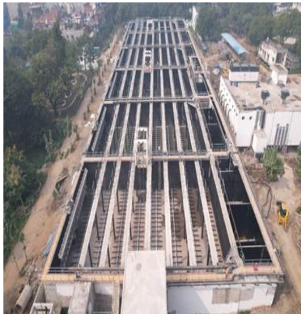
55 MLD STP at Assi BHU, Varanasi
