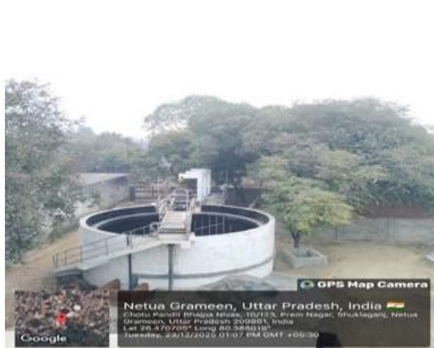
5 MLD STP at Shuklaganj
